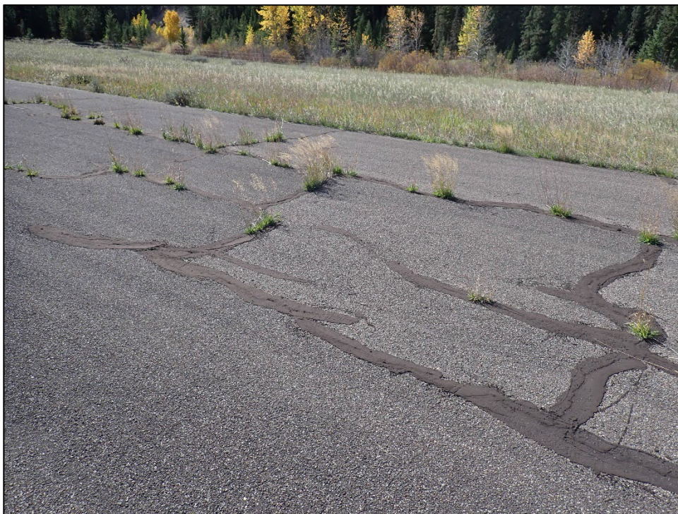
RW12-01-66: Block Cracking
