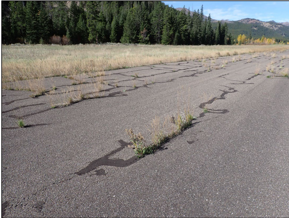
RW12-01-86: L&T Cracking
