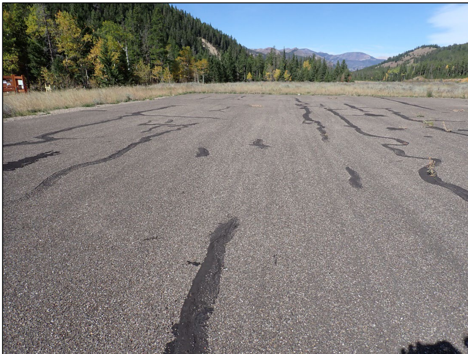
AP-01-07: L&T Cracking
