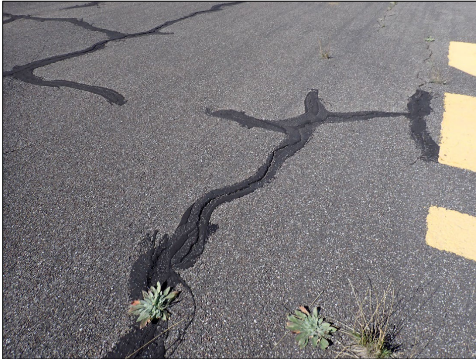
AP-01-05: L&T Cracking
